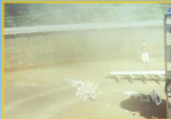
Cracks visible from outside of Clarifier
